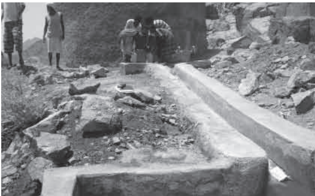
This water tank has a spill way. Excess water runs downhill into a section for livestock to drink from, away from the main water source.
