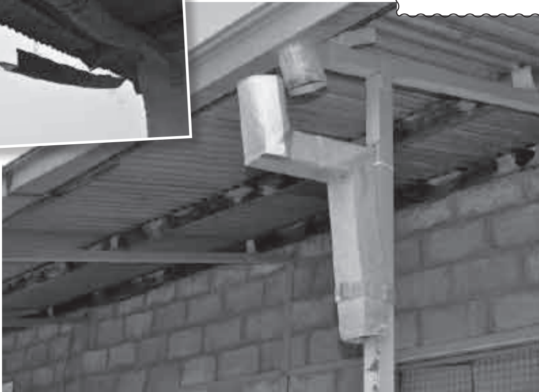
TOP: A simple invention to collect precious water. BOTTOM: Gutters need to be maintained or water will be lost.
